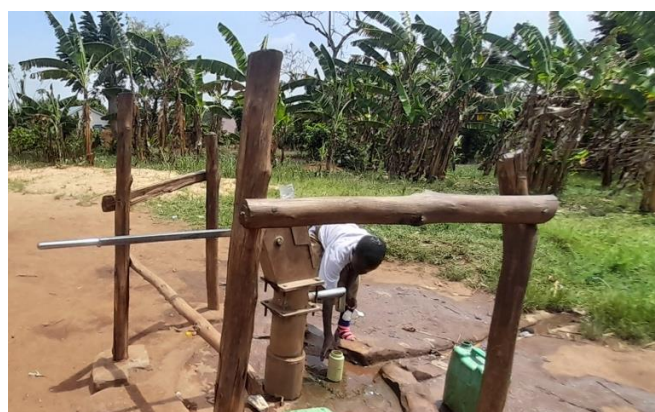
Figure 8: Water from a borehole with a pump
