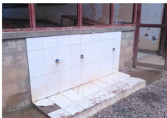
Figure 7: Public stand pipes with taps
